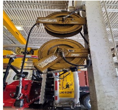
Bulk oil system — view 2
