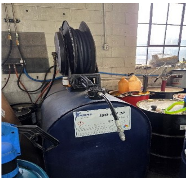
Bulk oil system — view 3
