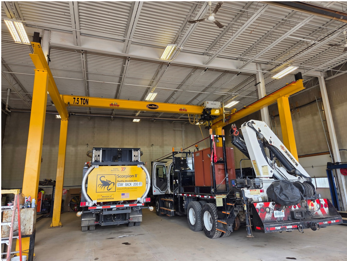
7.5-ton overhead bridge crane (29'6" span, installed 2015) spanning Bays 4 & 5
