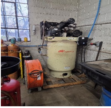
Ingersoll Rand air compressor Compressed air plumbed throughout shop.
