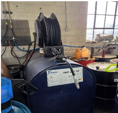
Bulk oil system — view 3
