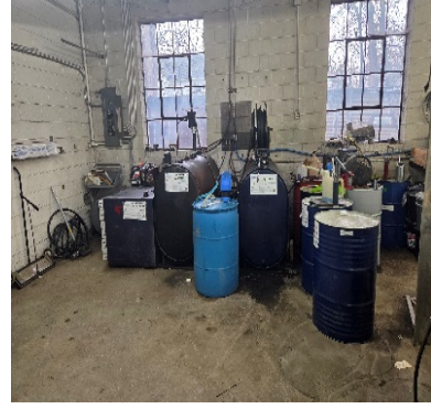
Bulk oil system — plumbed throughout shop Digital counter meters on every hose.
