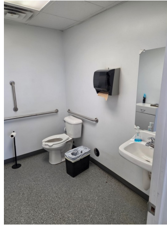
Customer restroom — code compliant
